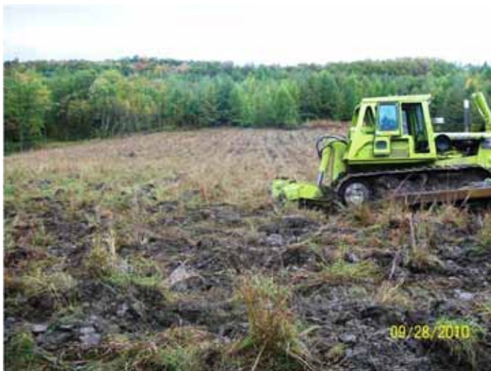
Ripping the soil to create favorable soil conditions for planting. Jeff Larkin
